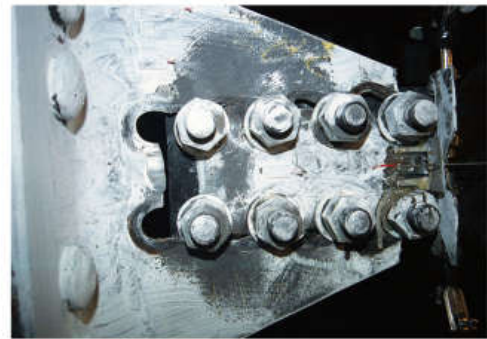
block shear fracture
