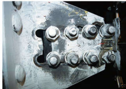
block shear fracture
