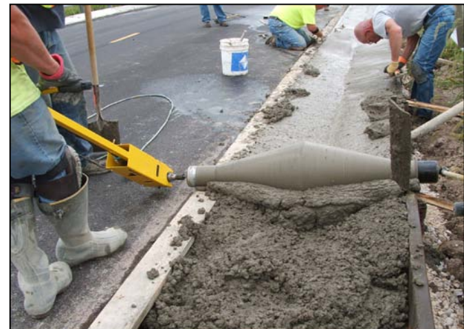
Spin Screed at work on an Illinois highway building a type A gutter
